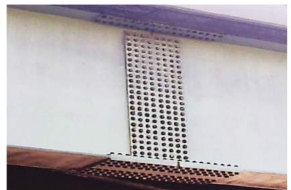
Typical splice plate joints used to connect the steel girders of a highway bridge.
